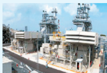
In-house turbine facilities at the Ichihara Works
