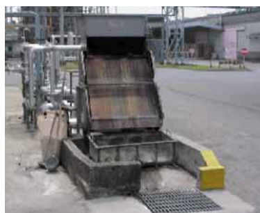
Strainer installation status (Ichihara Works)
