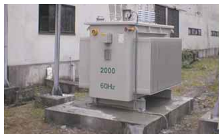
Installation status of amorphous transformers
