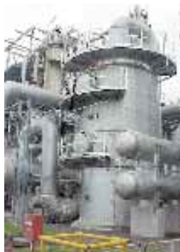
The exhaust gas catalyst oxidation unit
