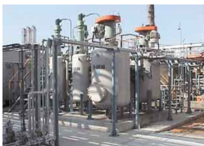
Ozone treatment unit (Ichihara Works)
